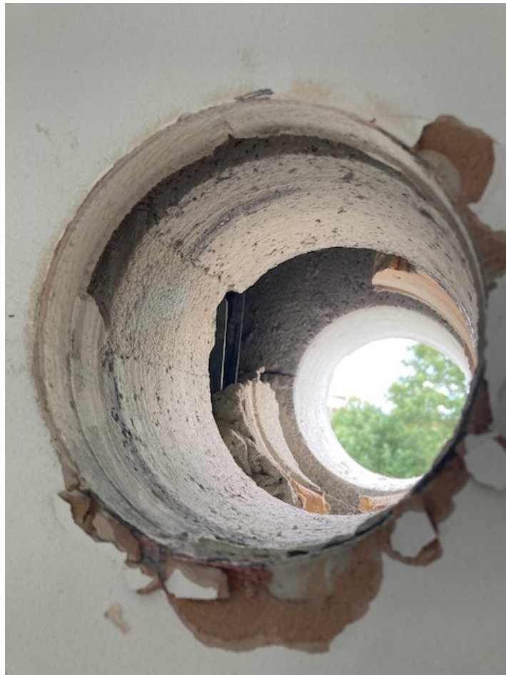
Photo 1- View through wall showing missing cavity insulation, poorly fitting insulation boards, gap between boards and inner leaf.
