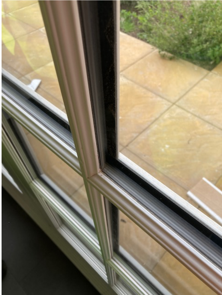
Photo 2- Basic double glazing with Georgian glazing bars, each spacer is a thermal bridge and reduces the performance of the pane, sash windows have poor long term airtightness
