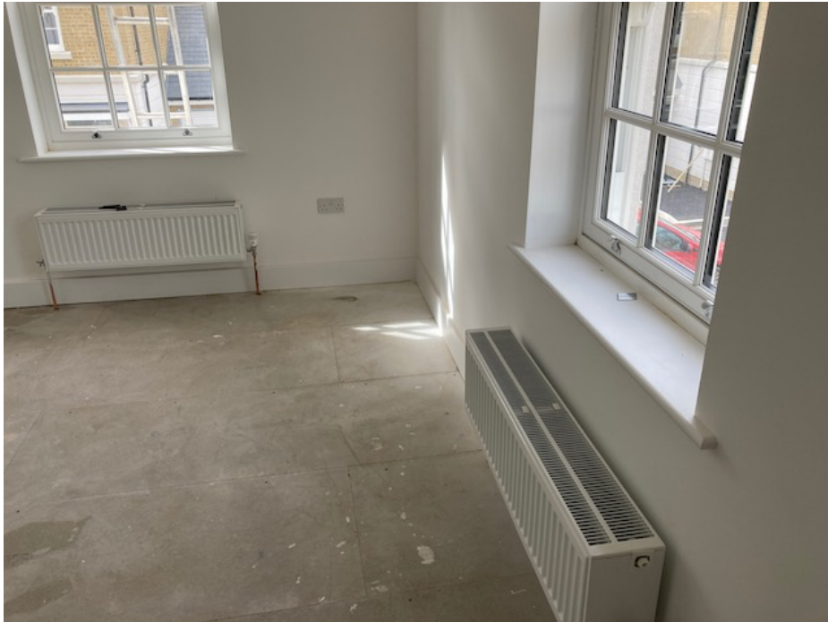
Photo 4- radiators did not need to be triples, it would be have been better to make them taller to avoid taking up floor space.
